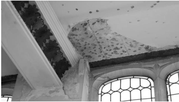
The ceiling of the library in Allen Hall is currently being restored
